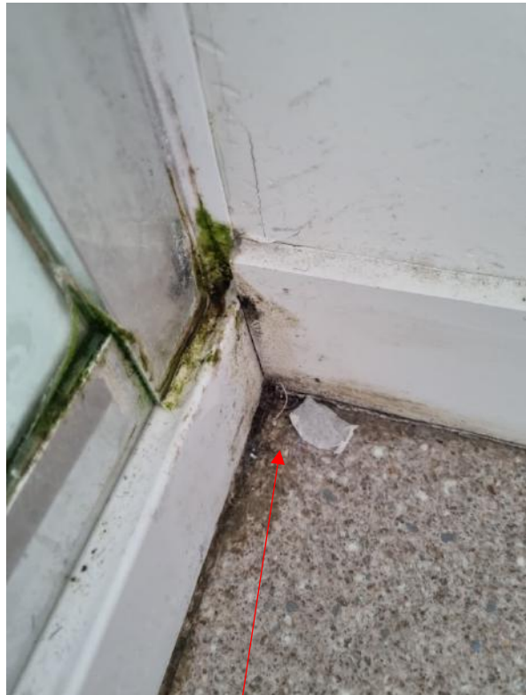
Shower showing excessive moisture – requires sealing
