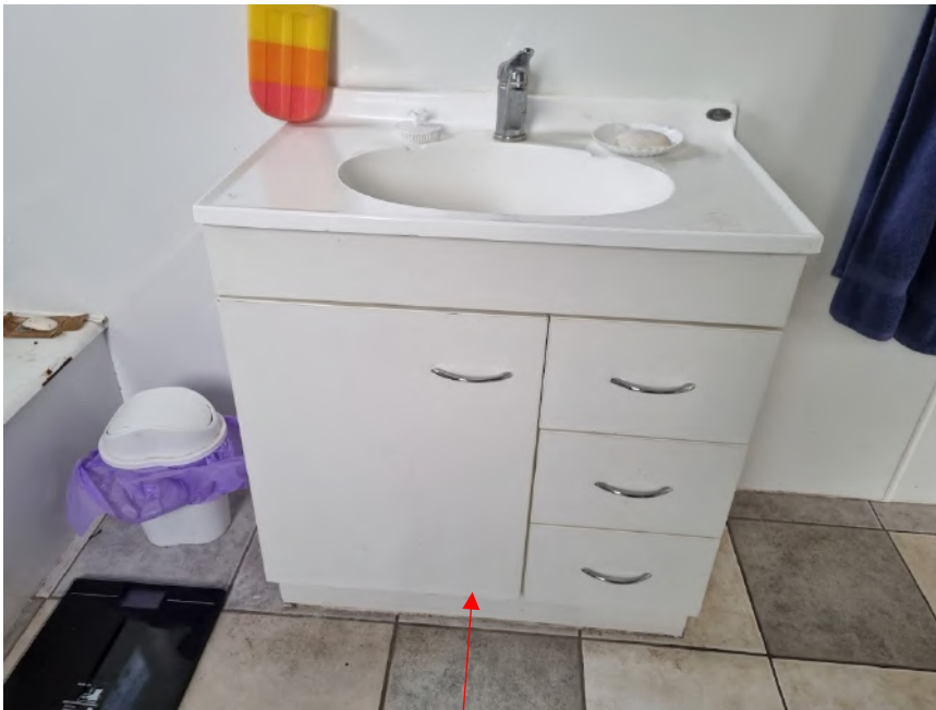
Vanity door in bathroom needs repair
