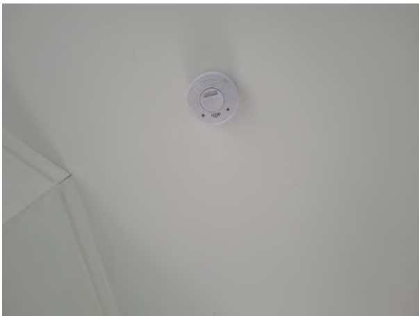
Smoke alarm present in Hallway
