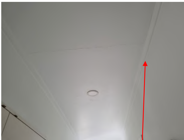
Hallway has surface crack in ceiling
