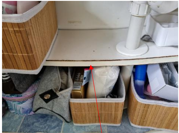
Vanity shelving in bathroom 2 is in poor condition
