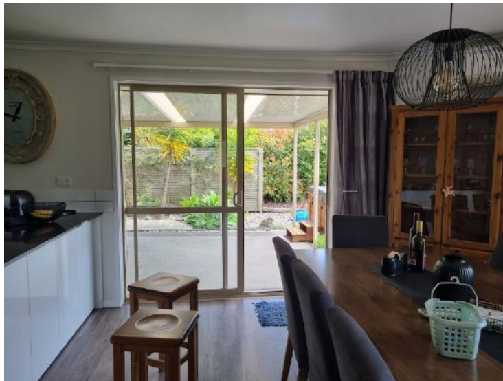
Missing Transition Bar
