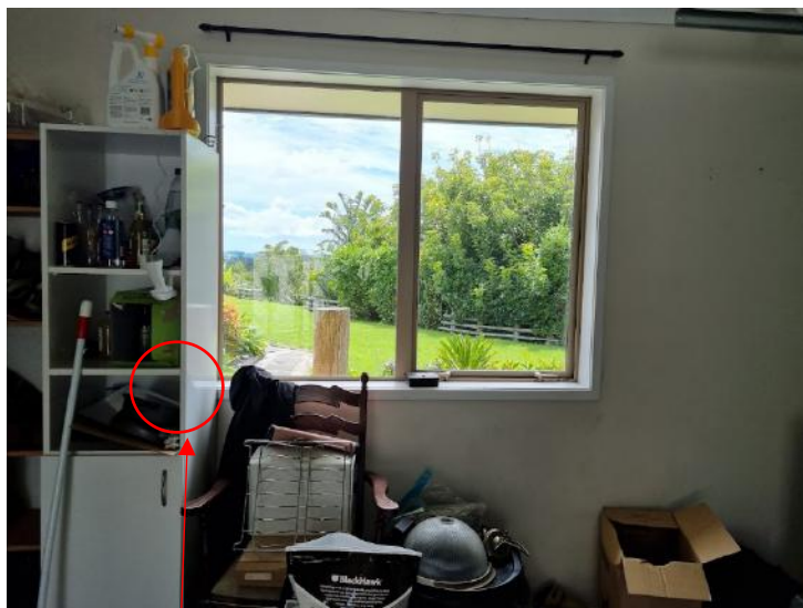
Cannot access left hand side of garage window due to cabinet blocking the moisture meter reading point.
