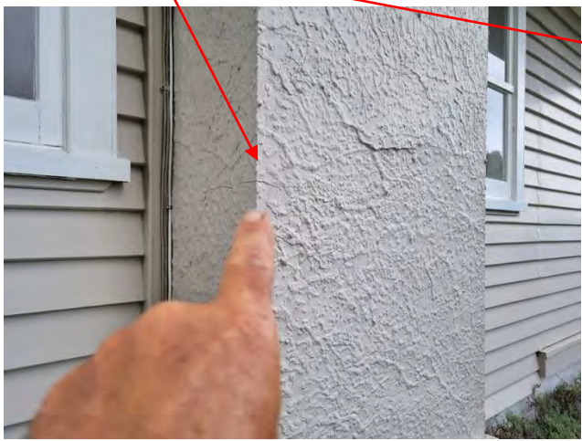
Chimney stack has a few cracks and further investigation required
